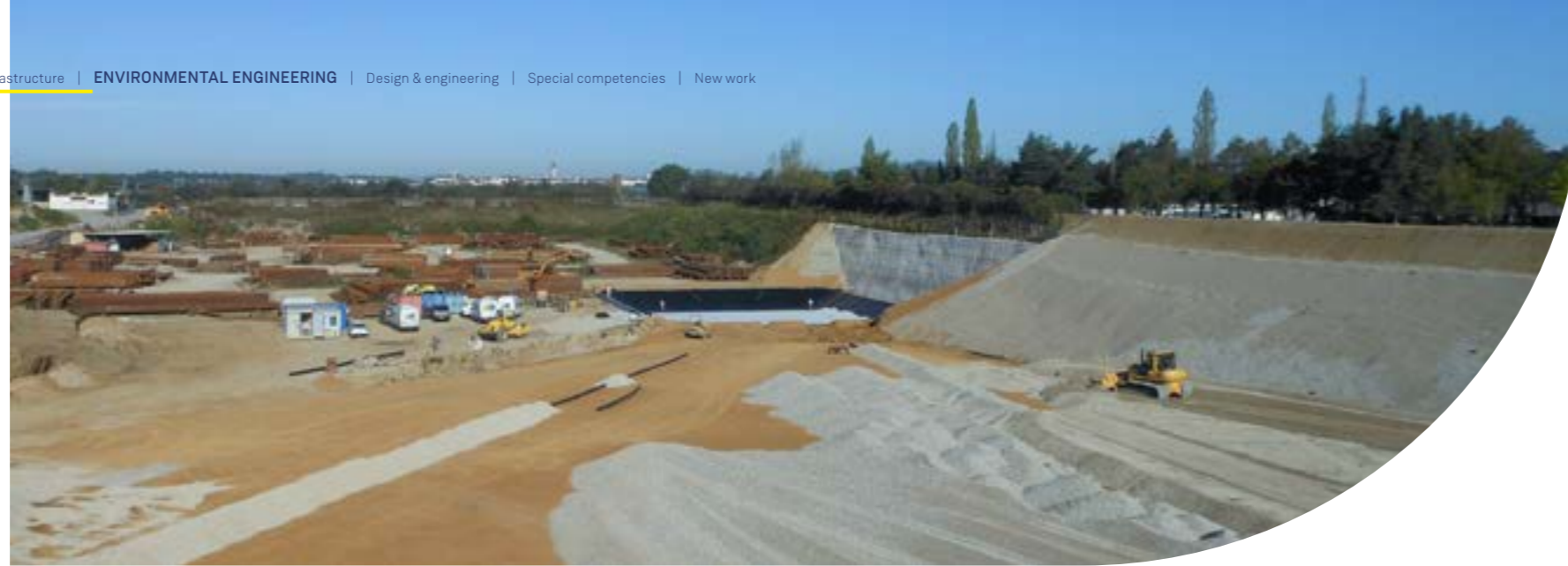
Rems construction waste landfill and recycling plant – Austria State-of-the-art storage for numerous types of waste
